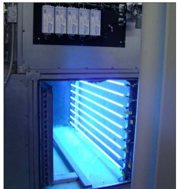
This application is intended to disinfect the air in one pass through the Air Handler. Due to the short duration of exposure to UV, there are nine bulbs. (Image: William P. Bahnfleth, ASHRAE UVGI Short Course)
